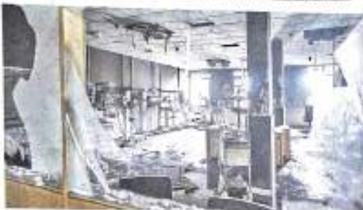
The charred remains of medical equipment after a fire ripped through the neonatal intensive care unit of a government hospital in Amravati district of Maharashtra on August 24. CHANAKYA NATOR
